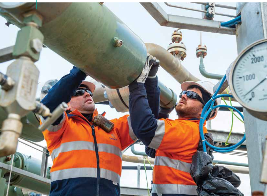
Ash Tregga and Cameron Lumsden, Maintenance Technicians at Otway Gas Plant, Victoria
