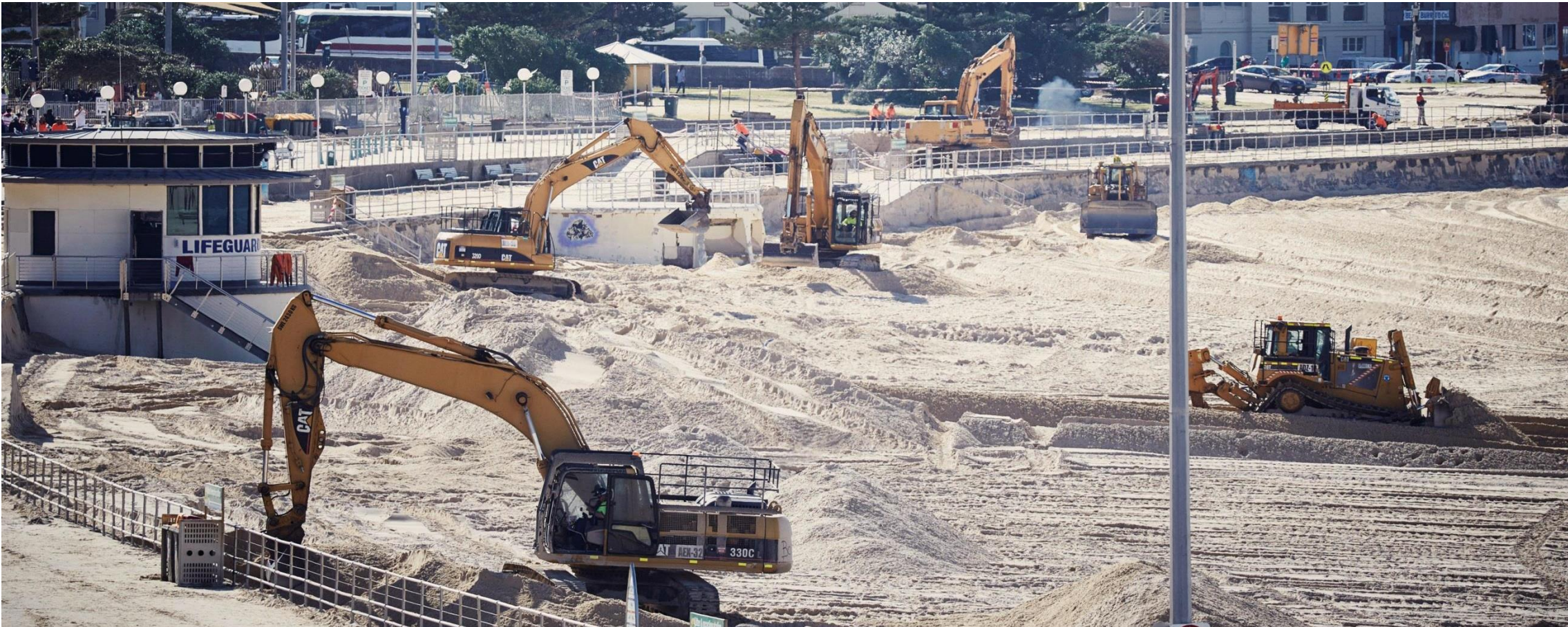
Cat excavators and dozers helped in the clean up effort after the severe storms in April 2015
