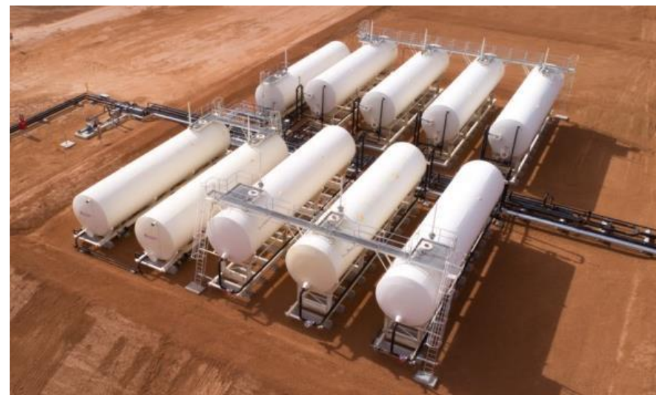
Bauer facility expansion (Cooper Basin), commissioned in Q4 FY17 Image: Beach Energy FY17 preliminary results presentation
