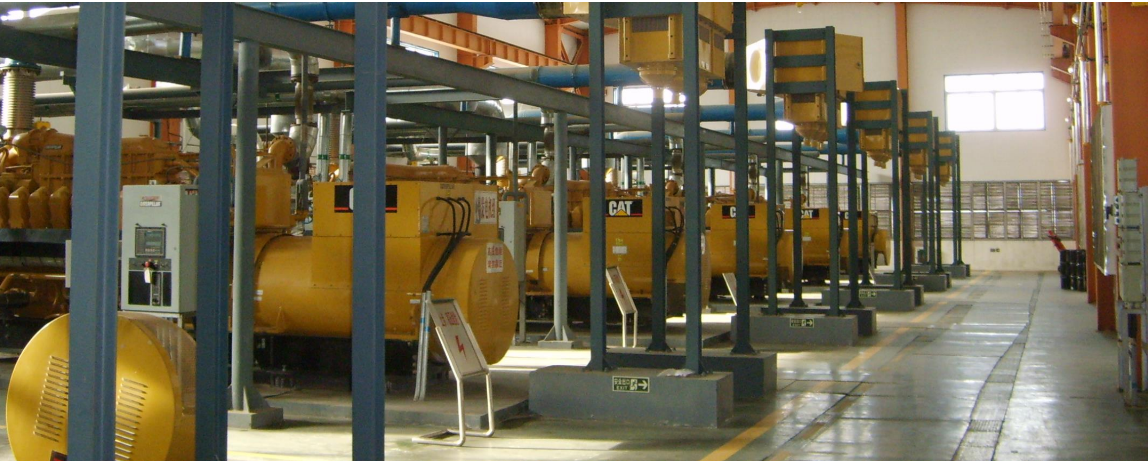
CAT generators provide backup power for a range of uses in the energy sector and data centres
