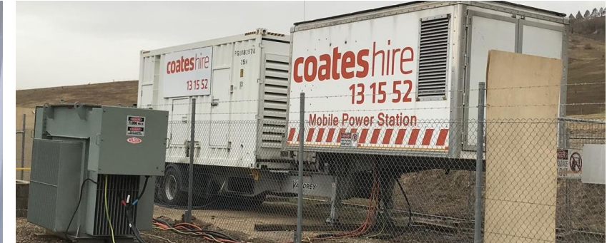
Genset deployed to Talbingo, NSW Snowy Mountains
