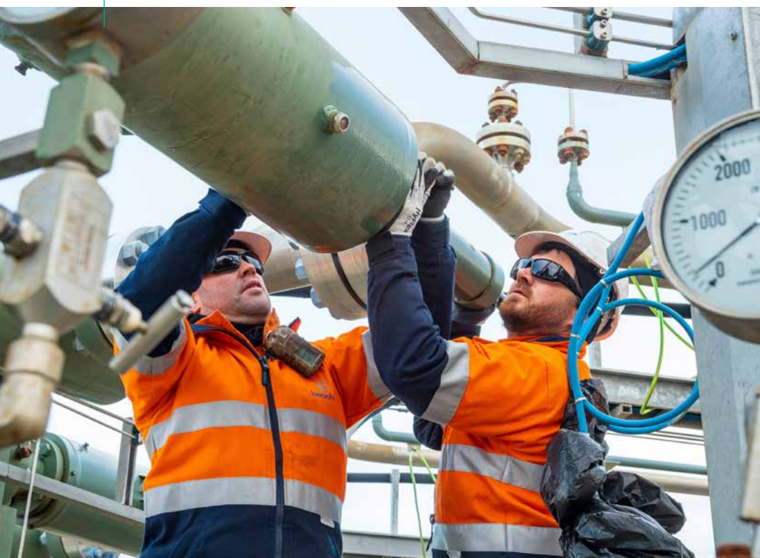
Ash Tregae and Cameron Lumsden, Maintenance Technicians at Otway Gas Plant, Victoria
