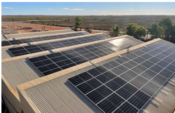
Newly installed Port Hedland solar panels
